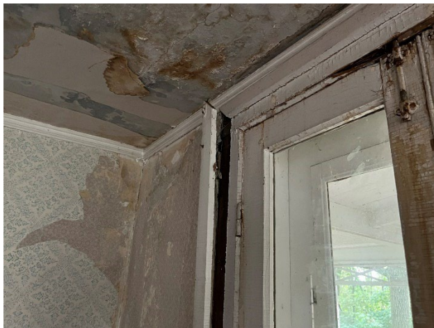
Figure 103. Water damage and deteriorated plaster wall.
