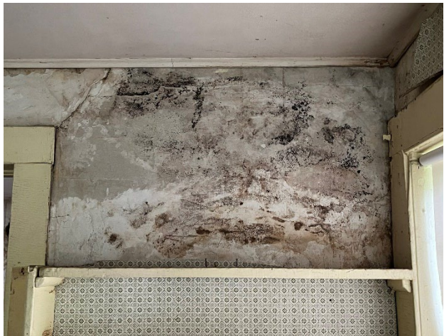
Figure 107. Biological growth on plaster at kitchen wall.
