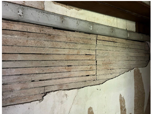
Figure 95. Missing plaster and exposed wood lath at wall.
