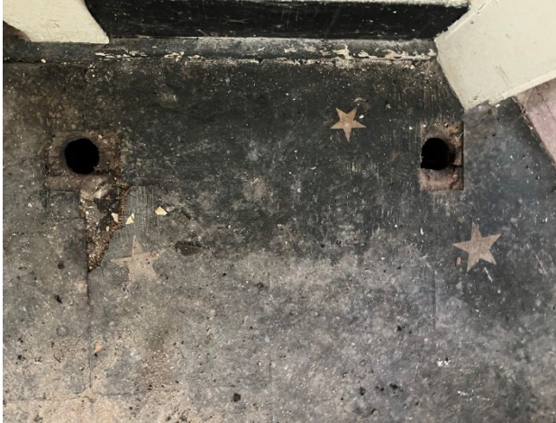
Figure 104. Water damage at second floor bathroom.
