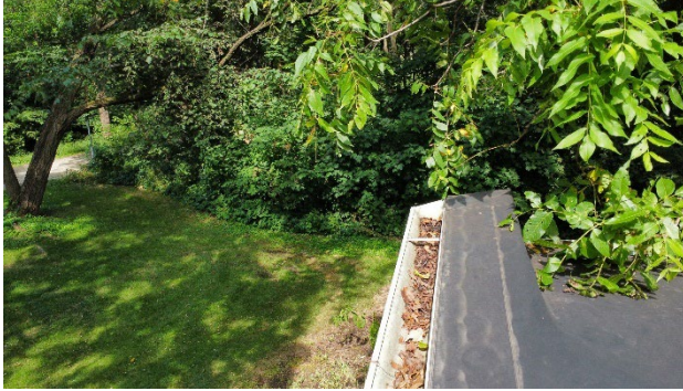
Figure 86. Miscellaneous debris in gutter at the southeast corner of the house.
