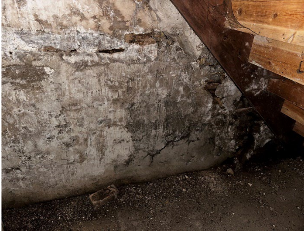
Figure 76. Water damage and efflorescence at interior masonry stone foundation wall.
