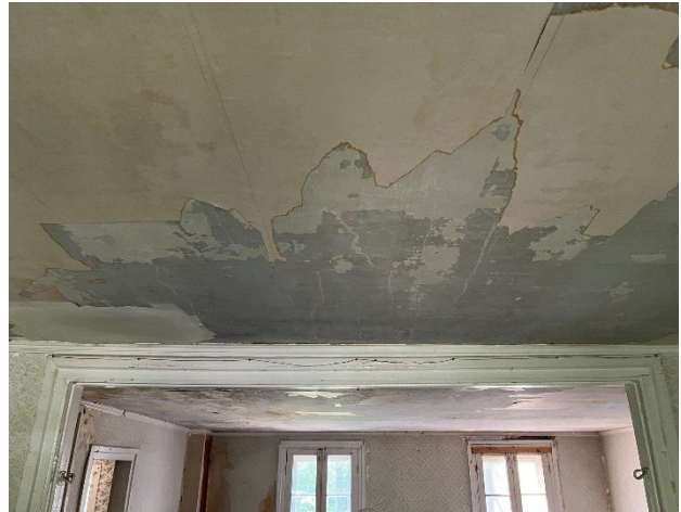
Figure 93. Cracked and deteriorated plaster at living room ceiling.
