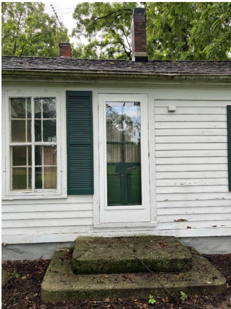
Figure 88. Paint failure at exterior wood components.
