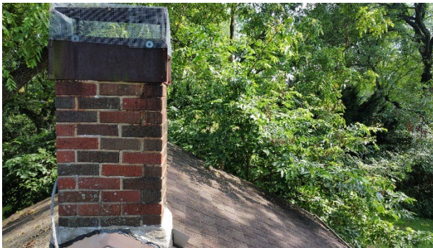
Figure 78. Minor masonry displacement at chimney over west wing.
