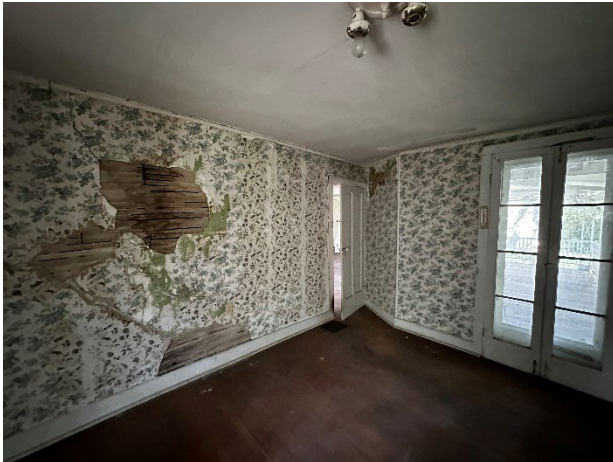
Figure 42. The east bedroom with doors leading to the front porch at right. An inspection opening was made as part of this study at the area of missing plaster at the left.
