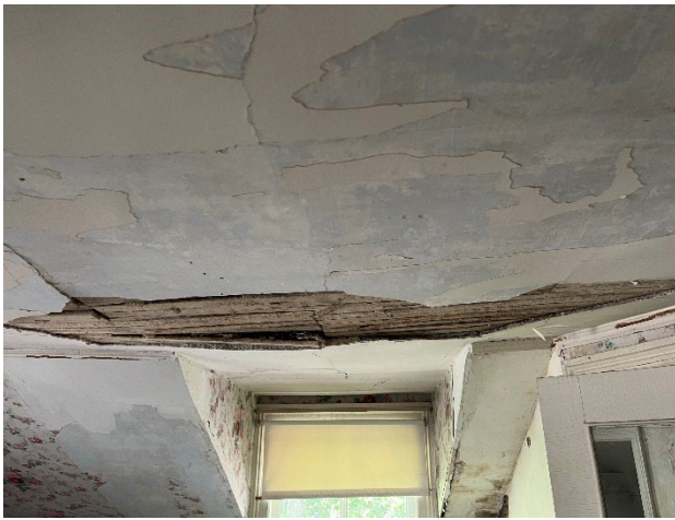
Figure 100. Damaged wood lath at plaster ceiling.
