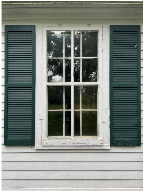
Figure 89. Paint failure at window framing.
