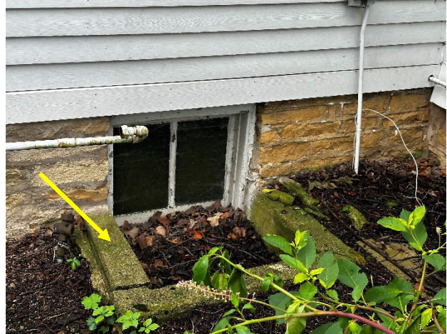
Figure 83. Biological growth on the concrete window wells (yellow arrow).
