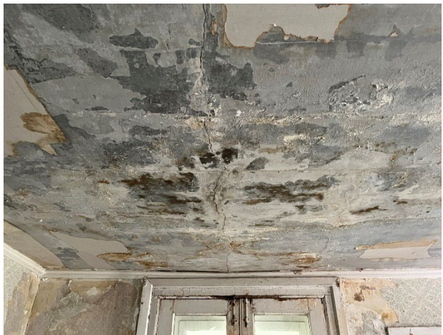
Figure 109. Biological growth at plaster ceiling in living room.
