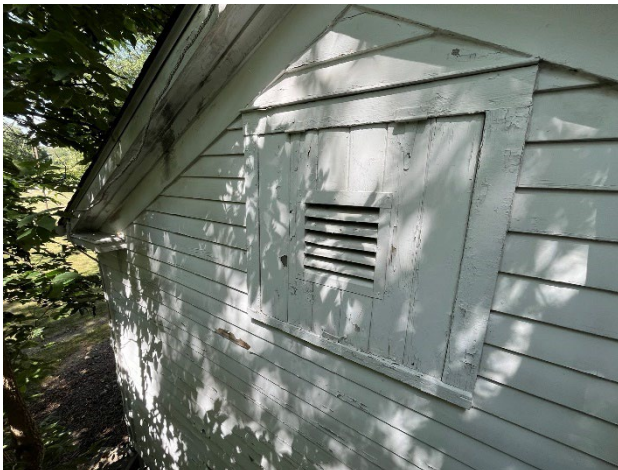
Figure 27. Partial view of south facade of the west wing showing the wood door with louver at the gable end.
