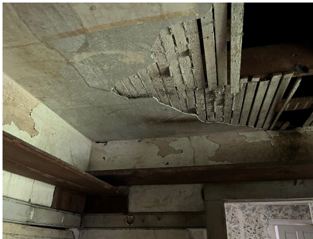
Figure 96. Cracked, deteriorated, and missing plaster at ceiling.
