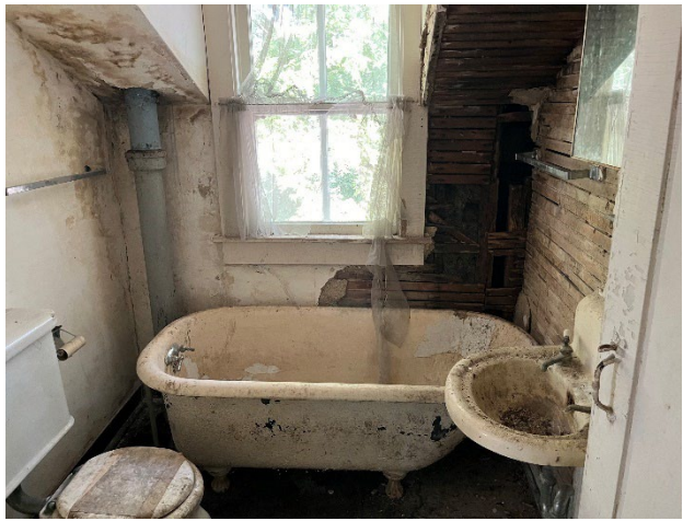
Figure 101. Extensive plaster damage and exposed wood lath at second floor bathroom.
