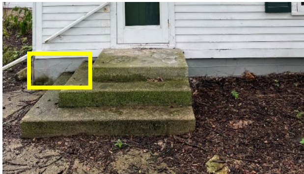
Figure 79. Biological growth and cracking at parge coat on west wing foundation (yellow box).
