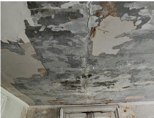
Figure 108. Biological growth at plaster ceiling in living room.
