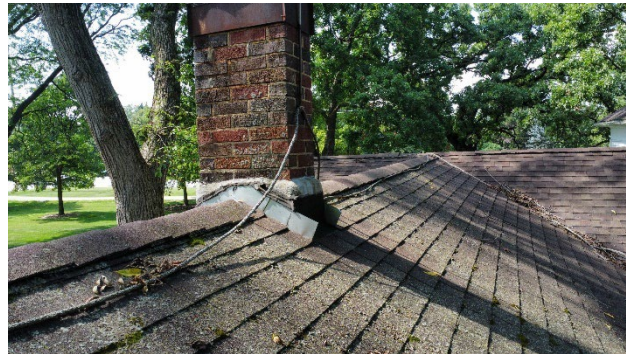
Figure 85. Biological growth on south side of west wing gable roof.
