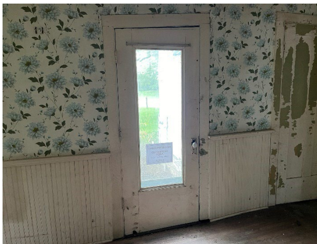
Figure 81. Evidence of past settlement at interior finishes in dining room.
