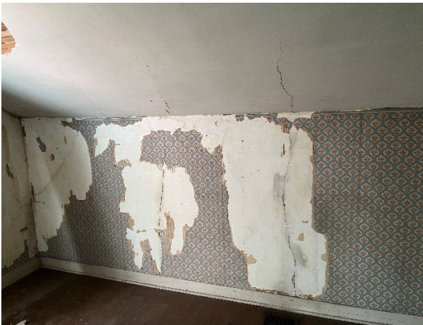
Figure 106. Peeled and missing wallpaper at cracked and damaged plaster at bedroom.
