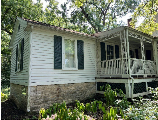
Figure 72. Step cracking in masonry mortar joints at northeast corner.
