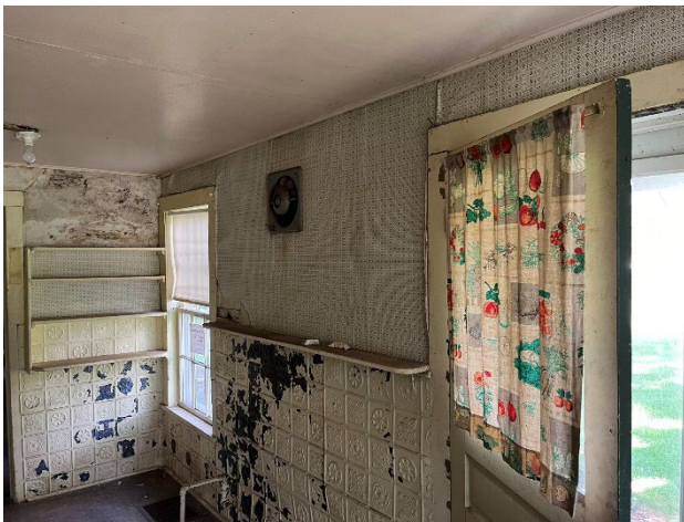
Figure 102. Peeling and flaking paint at interior finishes.
