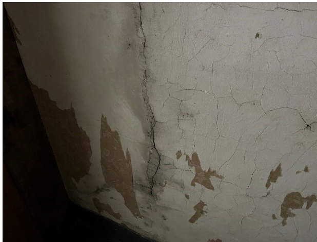
Figure 94. Cracked and deteriorated plaster at ceiling.
