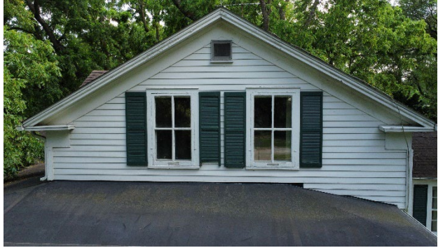
Figure 87. Biological growth on north roof over porch.
