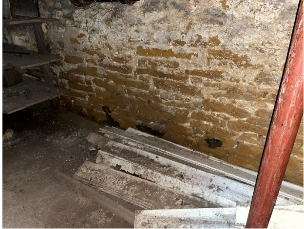
Figure 73. Deteriorated parge coat and open mortar joints at interior masonry stone foundation wall.
