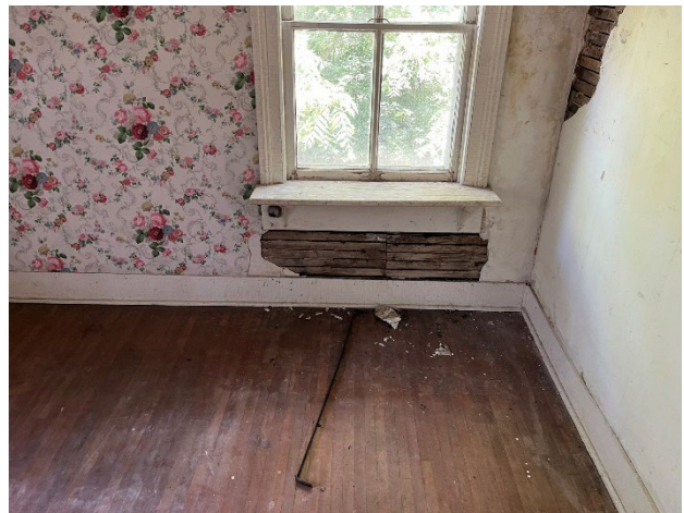
Figure 97. Cracked, deteriorated, and missing plaster at front bedroom wall.
