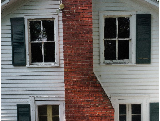
Figure 77. Deteriorated mortar joints at chimney on south wall.
