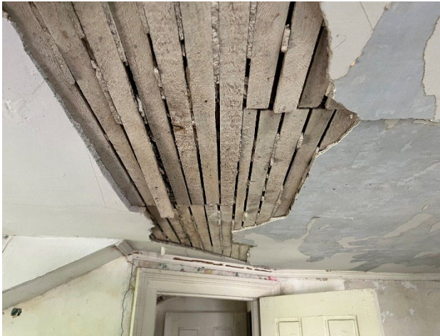
Figure 98. Cracked, deteriorated, and missing plaster at front bedroom ceiling.
