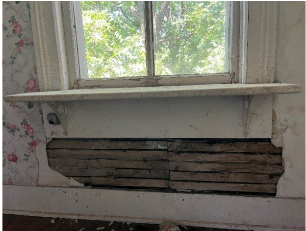
Figure 99. Missing plaster and exposed wood lath.
