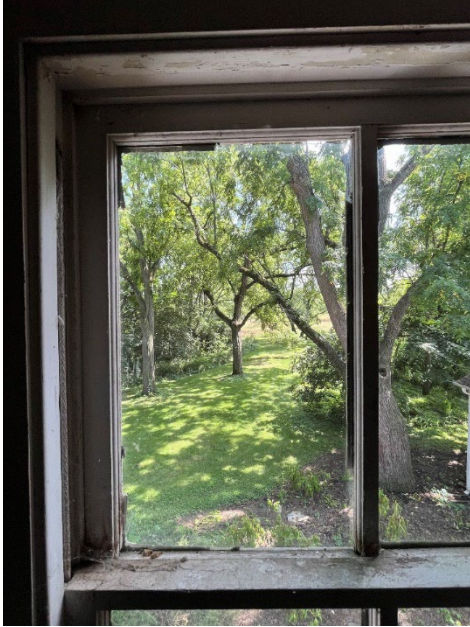
Figure 90. Deterioration of window glazing putty at second floor windows.
