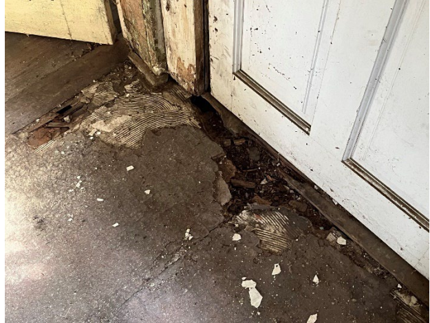
Figure 105. Water damage and deterioration at floor. Of second floor bathroom.
