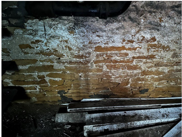
Figure 75. Open mortar joints at interior masonry stone foundation wall.
