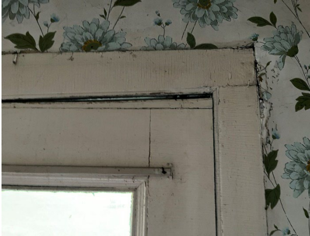
Figure 82. Evidence of movement and displacement at door frame in dining room
