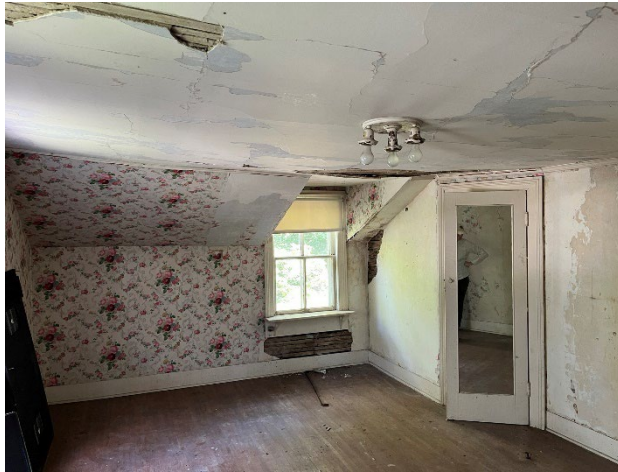
Figure 92. Cracked and deteriorated plaster at front bedroom ceiling.
