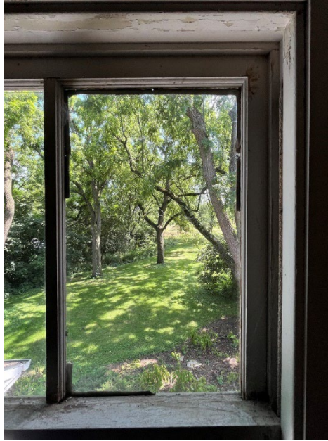
Figure 91. Deterioration of window glazing putty at second floor windows.
